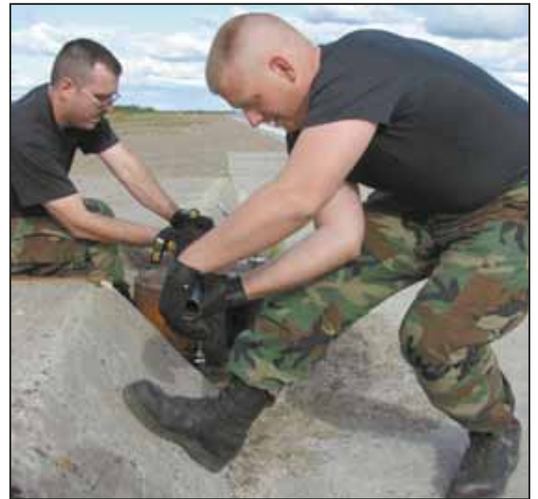
Courtesy photo/Tommie Baker, U.S. Air Force Master Sgt. Troy Snipes, left, steadies a breaker bar for Staff Sgt. James McCormick. Both men are 611th Civil Engineer Squadron power production craftsmen assigned to Elmendorf Air Force Base. Snipes and McCormick are on temporary duty to Galena Airport to disassemble and remove three sets of barrier arresting kits. The BAK-12s, the standard emergency aircraft-arresting system in service with the U.S. Air Force, were used over the years to help stop distressed fighter aircraft as they landed at the airfield. Galena Airport, used as a forward operating location for the Air Force, will cease all military operations by Sept. 30, 2008, as part of recommendations by the 2005 Base Realignment and Closure Commission.
